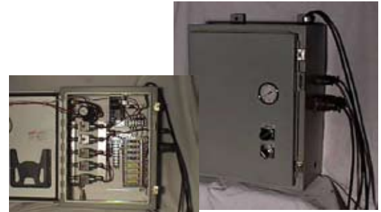
VALVE CONTROL BOX
